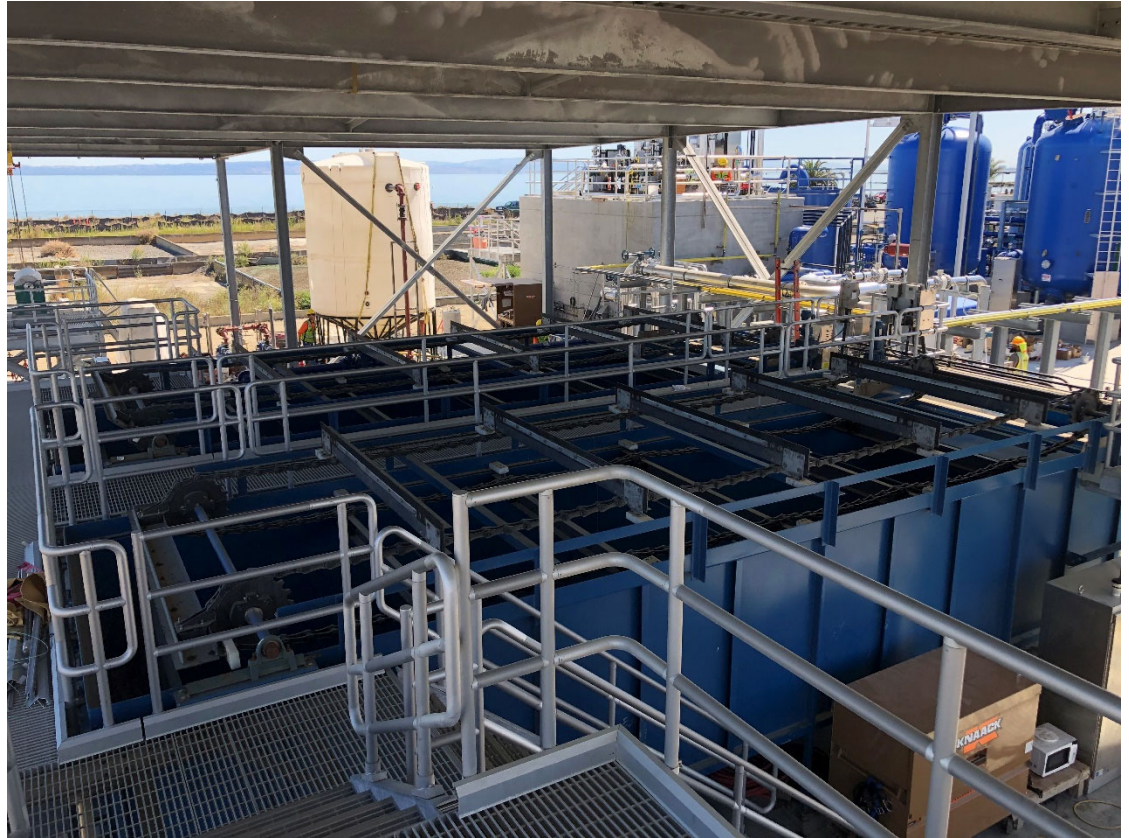
Figure 7.6 DAF Unit Sludge Scraper System
