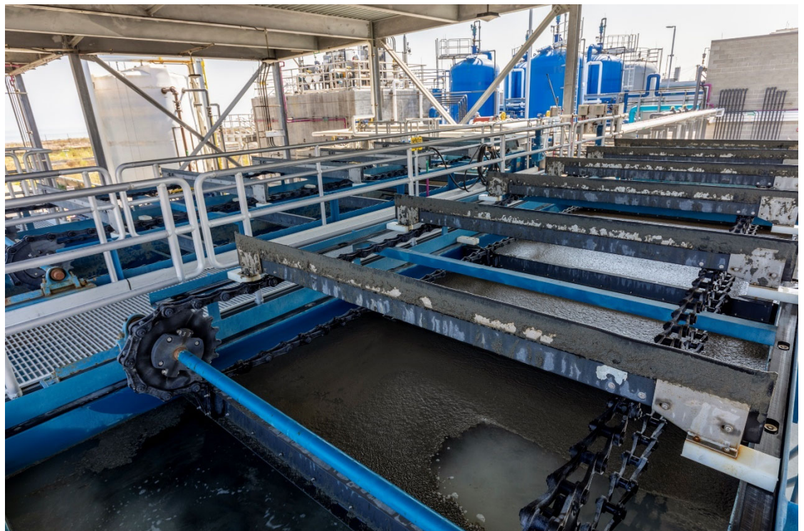
Figure 7.7 DAF Unit in Service
