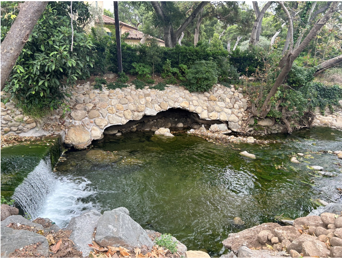
Photo 2: Site area after erosion
