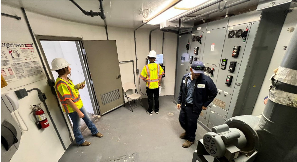
WSC staff met with MSD operations staff as part of a field investigation effort for the MSD-SSD intertie project. In the photo above, WSC and MSD staff were confirming pump sizes and capacity at the Posilipo lift station site. Results helped inform costs for intertie infrastructure alternatives.
