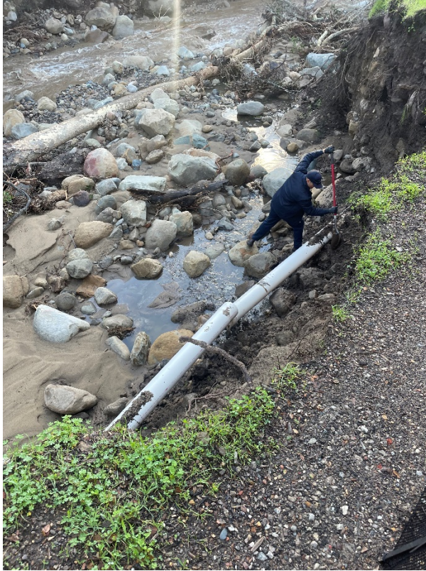
Photo 4: After Storm Pipe Break
