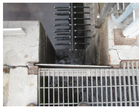
Photo 3.24 Aeration Basin 2 Channel Gate
