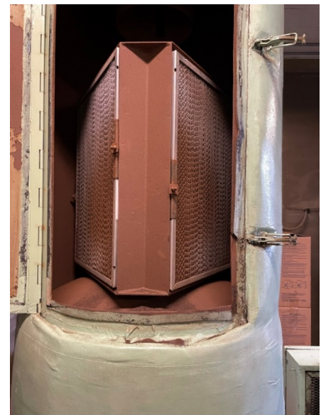
Photo 3.32 Aeration Basin Filter Silencer
