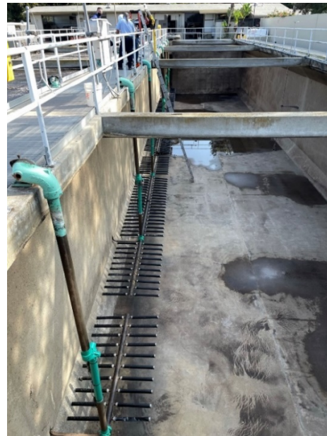
Photo 3.26 Air Diffuser System
