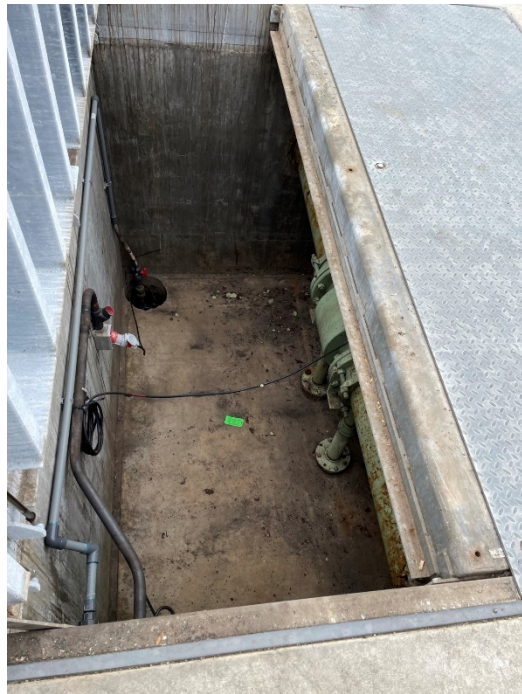
Photo 3.15 Influent Meter Vault
