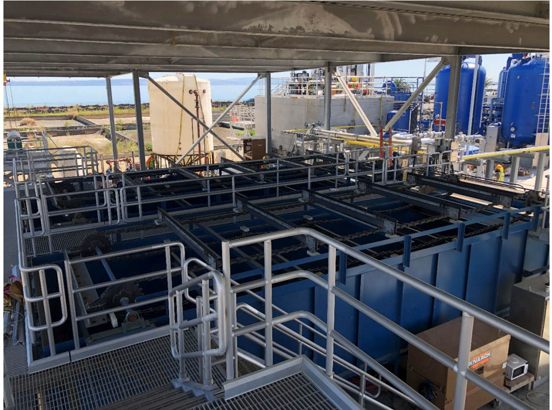
Figure 7.6 DAF Unit Sludge Scraper System
