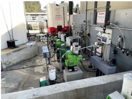
Photo 3.35 Sodium Hypochlorite Storage Facility
