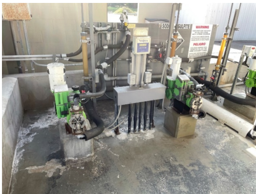
Photo 3.36 Sodium Bisulfite Storage Facility
