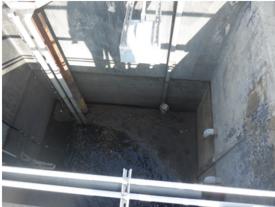
Photo 3.39 RAS/WAS Wet Well
