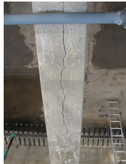
Photo 3.20 Aeration Basin 2 Cross Beam Longitudinal Cracking
