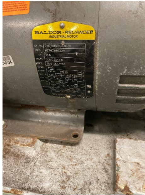
Photo 3.10 IPS Pump Room (Equipment Baseplate)
