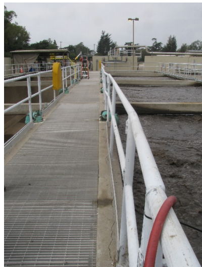
Photo 3.19 Aeration Basin Cracking at Guard Post
