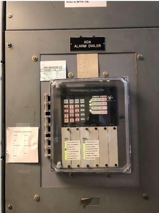
Photo 3.49 Old Control and ADA Alarm Panel
