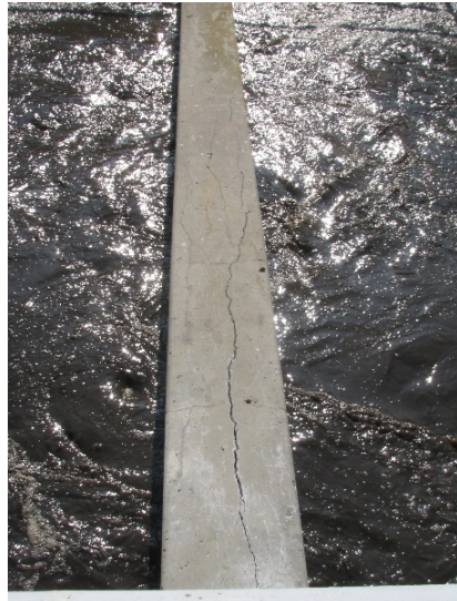
Photo 3.17 Aeration Basin 1 Strut Cracking
