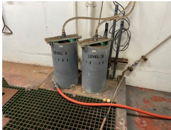
Photo 3.7 Wet Well Levels
