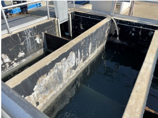
Photo 3.33 Chlorine Contact Basins
