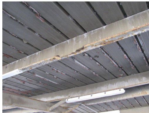
Photo 3.38 Sodium Hypochlorite Storage Facility Canopy
