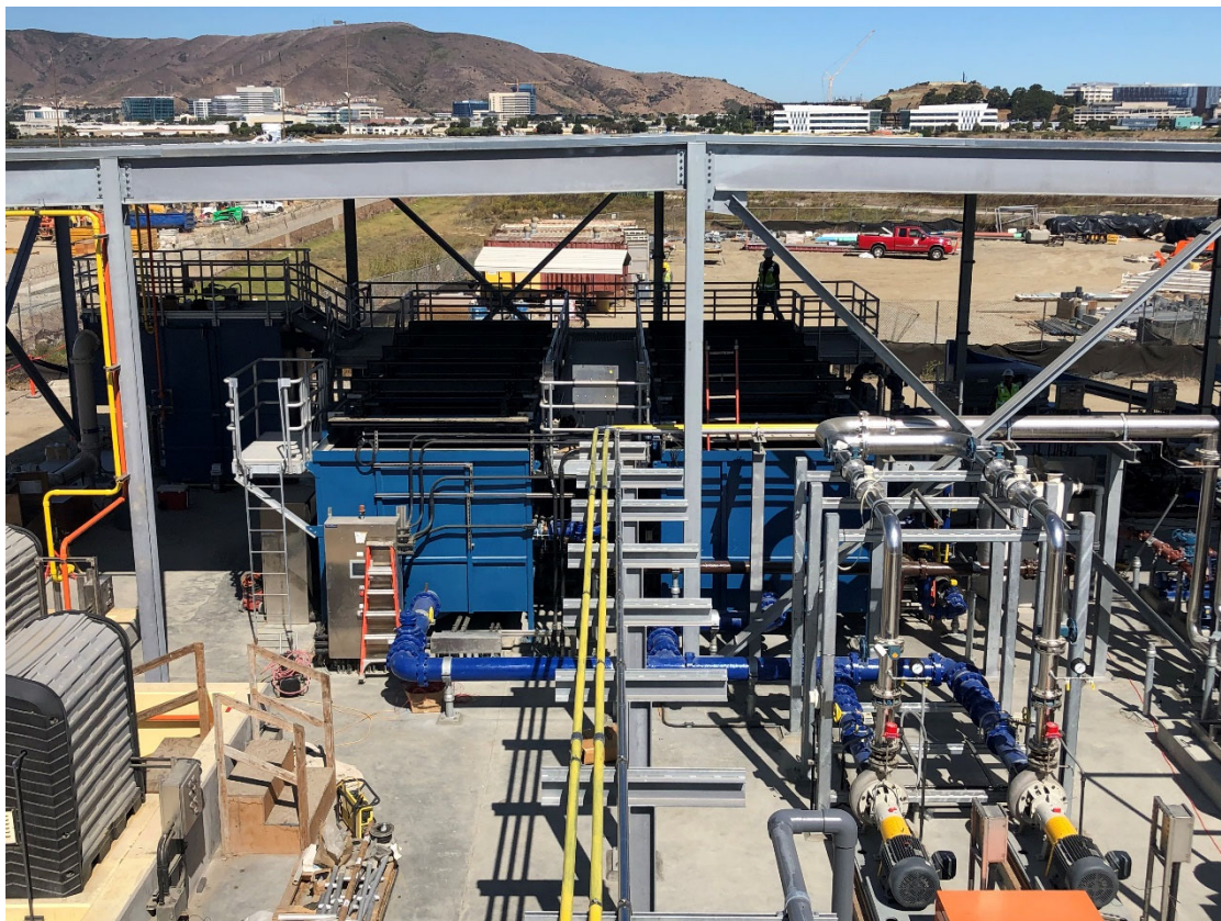
Figure 7.5 DAF Unit Contact Basin with External Platform and Chemical Feed System
