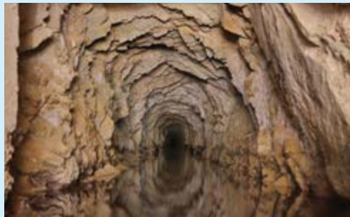
Doulton Tunnel, a horizontal well, source of groundwater and conveyance from Jameson Lake.
