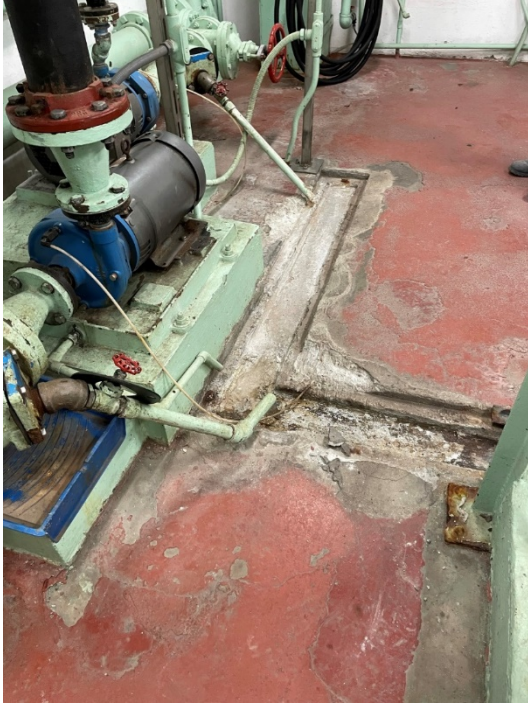
Photo 3.9 IPS Pump Room (Intermediate Level)
