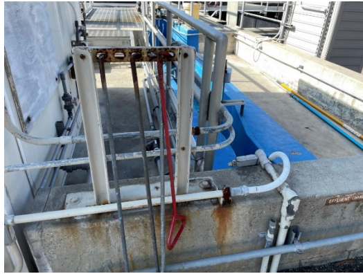
Photo 3.34 Chlorine Contact Basin Mechanical Equipment
