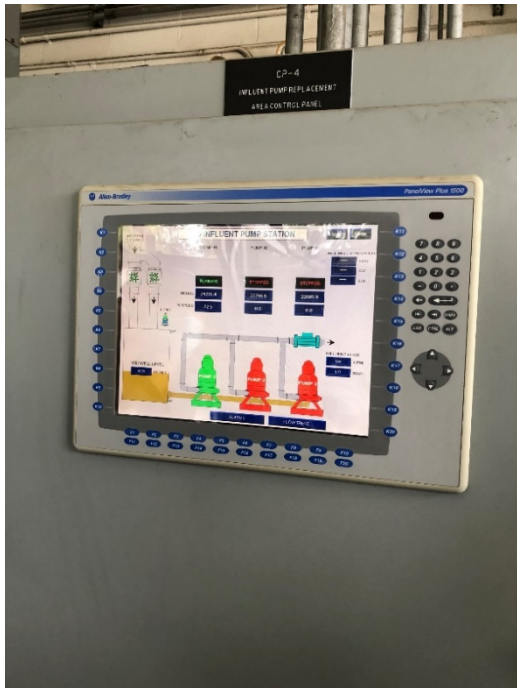
Photo 3.11 IPS Control Panel
