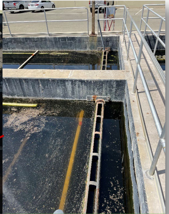
Clarifier Scum Trough (4)
