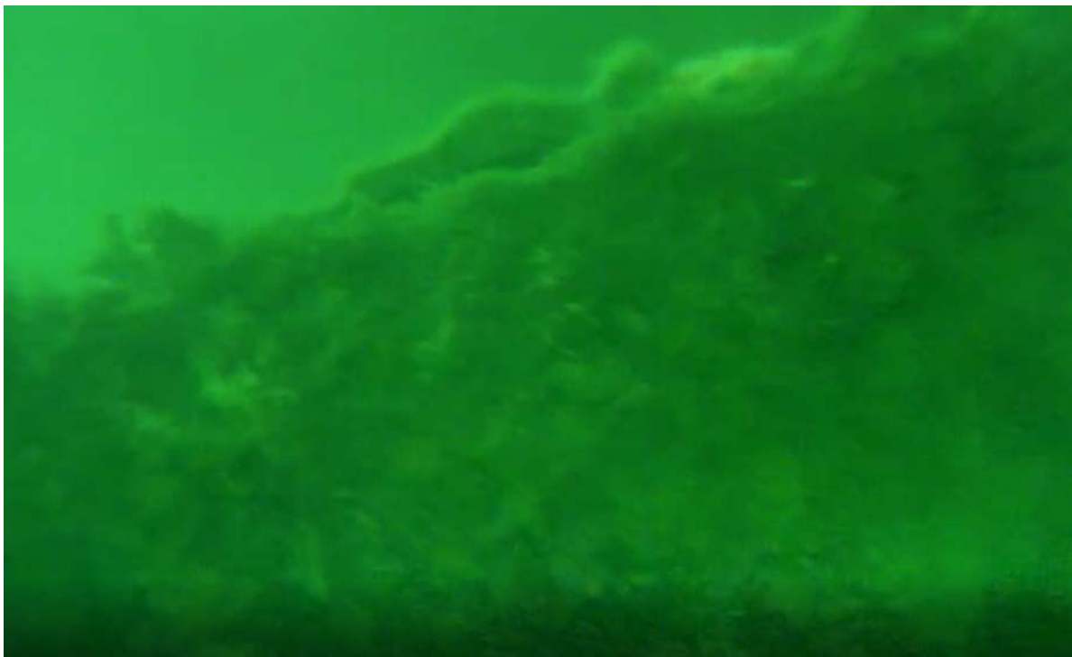
Opening in the top of diffuser 6
