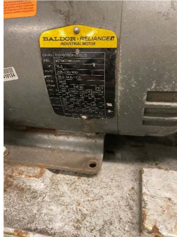
IPS Pump Room Baseplate
