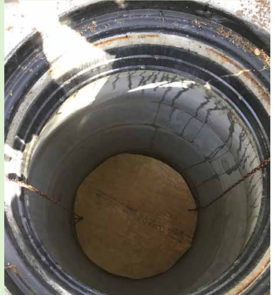
The plywood sits on the manhole concrete shelf which allows sewer to continue flow to the next pipeline.
