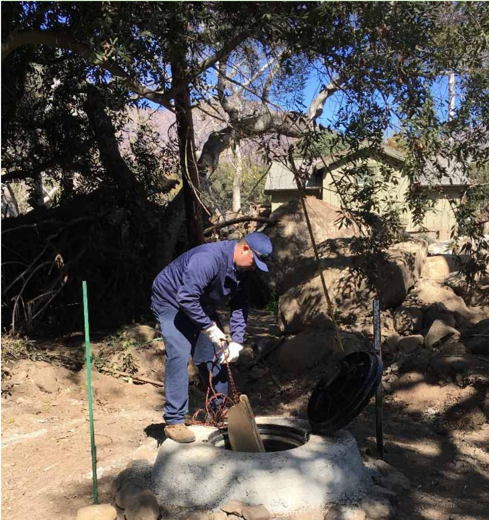
Protectors can be lowered by one person without having to enter the manhole.
