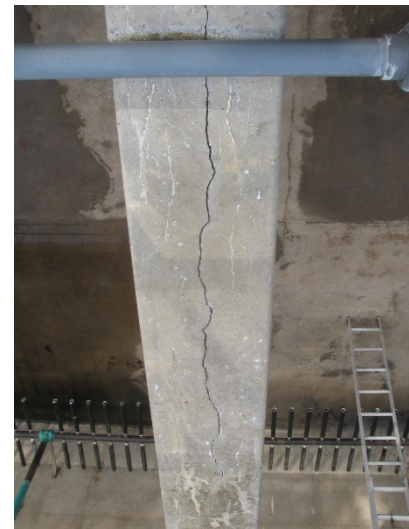
Photo 3.20 Aeration Basin 2 Cross Beam Longitudinal Cracking
