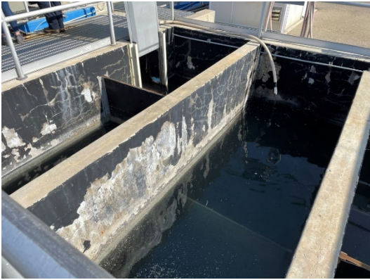
Photo 3.33 Chlorine Contact Basins
