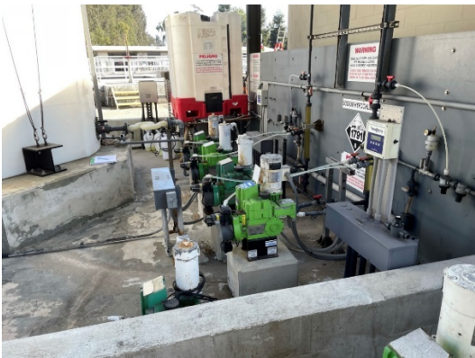
Photo 3.35 Sodium Hypochlorite Storage Facility
