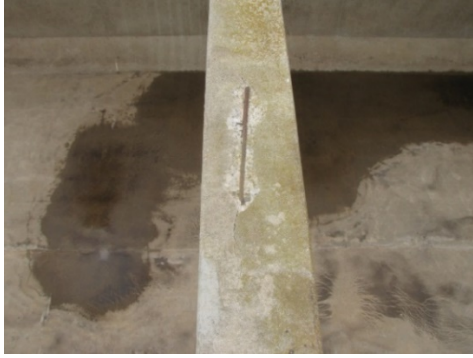
Photo 3.21 Aeration Basin 2 Exposed Rebar
