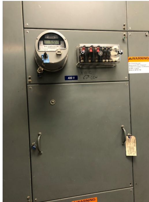
Photo 3.50 Service and Metering Cabinet
