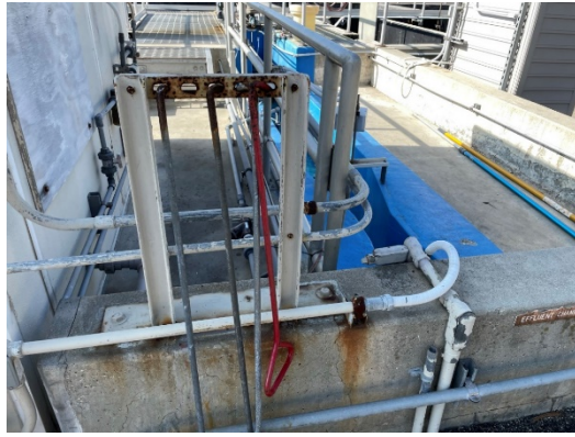
Photo 3.34 Chlorine Contact Basin Mechanical Equipment
