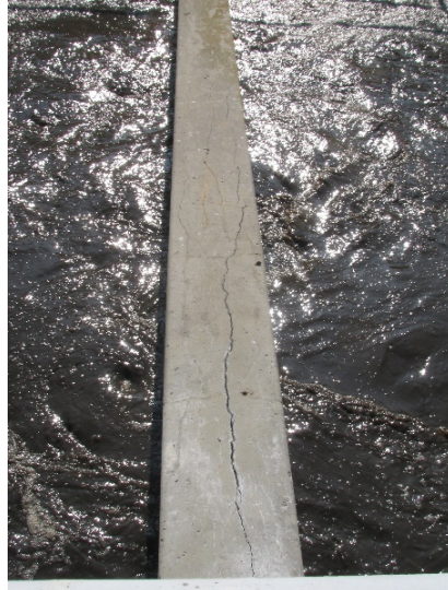
Photo 3.17 Aeration Basin 1 Strut Cracking
