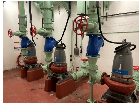
Photo 3.8 Influent Pumps/IPS Pump Room (Basement Level)
