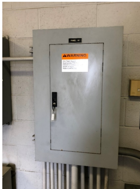
Photo 3.44 Blower Room Distribution Panels
