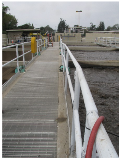
Photo 3.19 Aeration Basin Cracking at Guard Post
