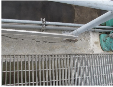
Photo 3.22 Aeration Basin 2 Evidence of Repairs
