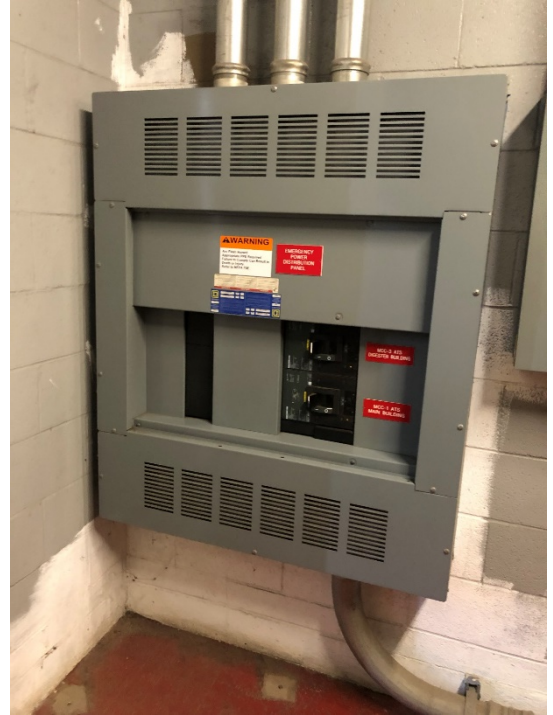
Photo 3.14 Emergency Distribution Panel
