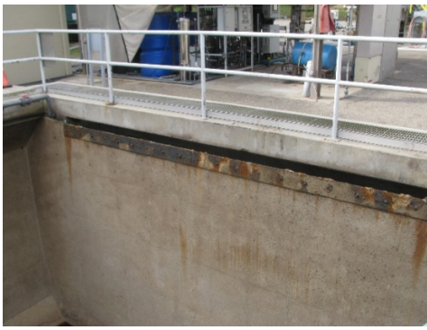
Photo 3.23 Aeration Basin 2 Wier Plate
