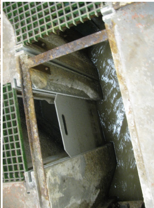
Photo 3.4 Influent Stop Plate
