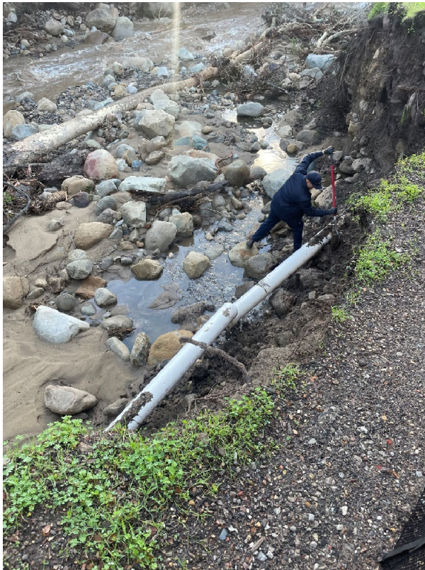
Photo 7: After Storm Pipe Break
